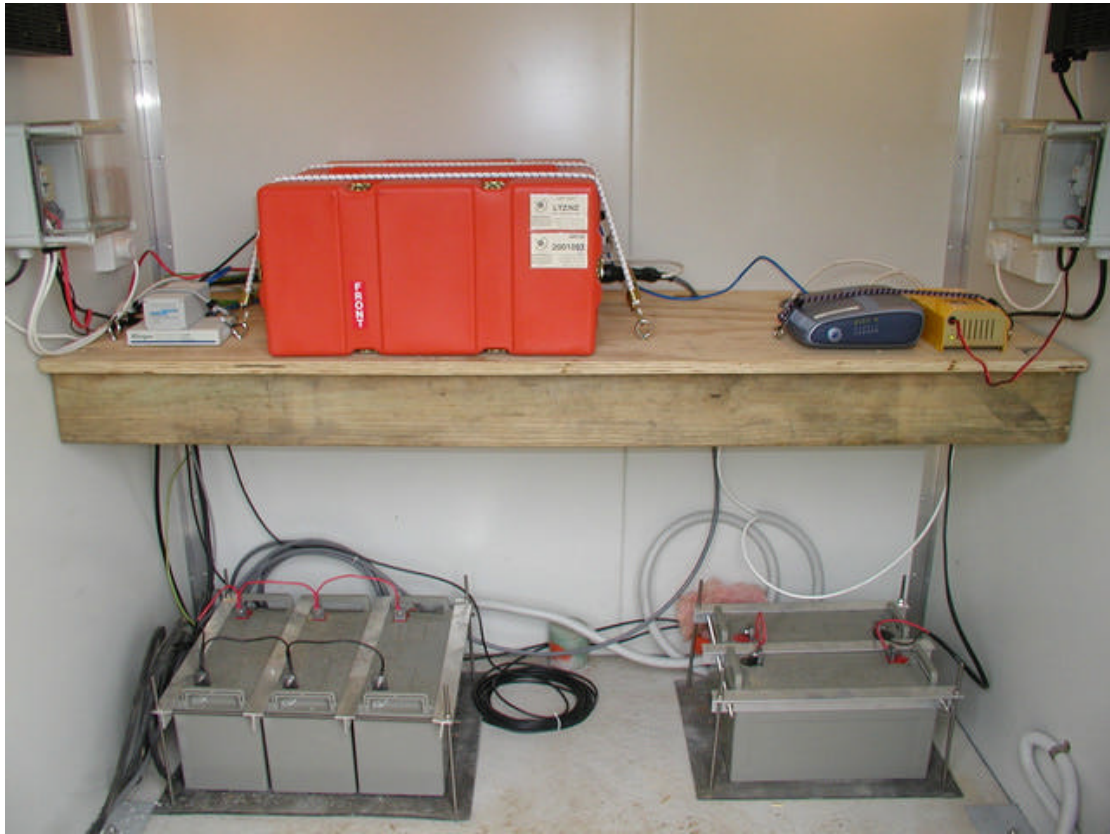
Figure 4.A photograph of the inside of a NZNSN equipment hut showing the orange Quanterra Q4120 to the left and the VSAT indoor unit to the right on the bench. The digitiser and VSAT communications equipment have separate power supplies with backup batteries on the floor of the hut. This site also records the data from a CGPS station (using a Trimble NetRS) via a Freewave Ethernet Bridge radio to the left of the Quanterra.
